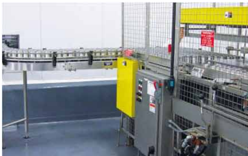
Crate loader places cans into crates to be retorted. A similar unit removes the cans.
